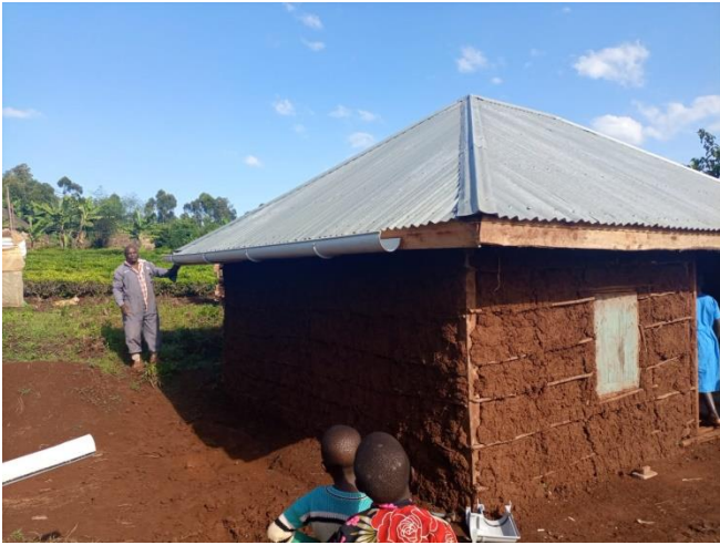
Gravity Feed with Water Tank on Pastor Erick's Home
