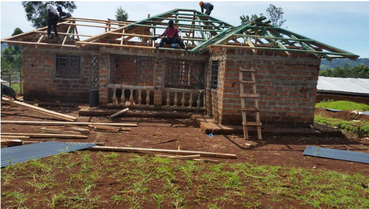
Rafters to support a new metal roof that will eventually carry rain gutters for water tank
